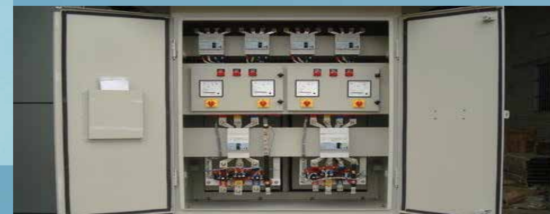
FEEDER PANEL BOX
